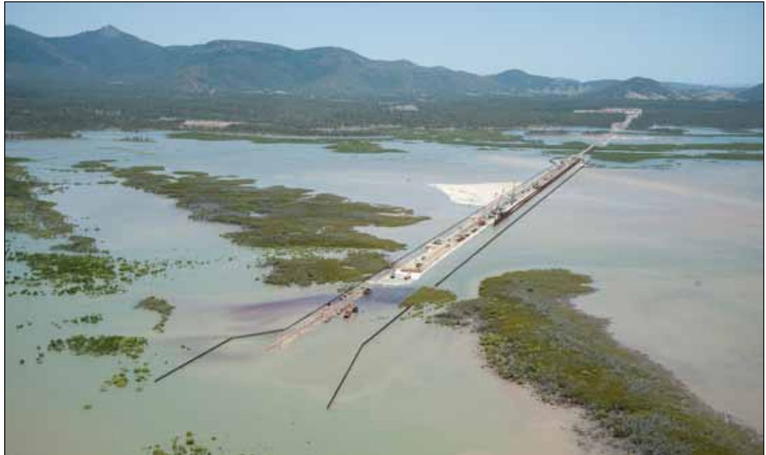
► Laying the pipeline which will supply CBM to the Queensland Curtis LNG plant on Curtis Island.
