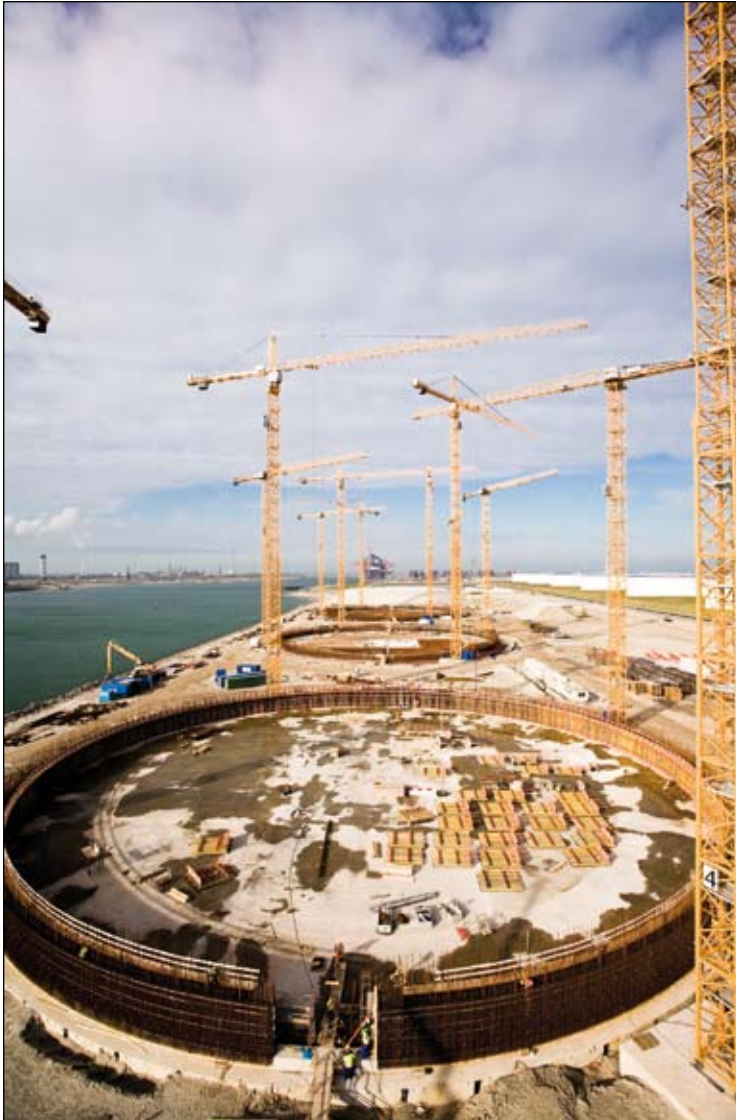
Gate in Rotterdam is the first LNG import terminal to be built in The Netherlands.
