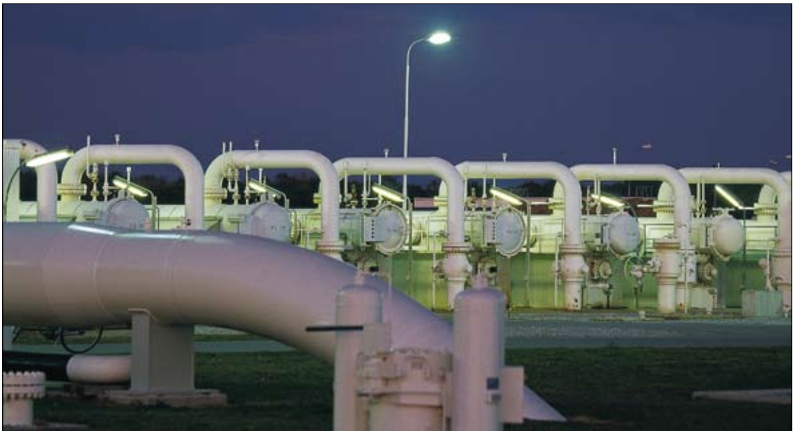
TOP Sources of gas for the Nabucco pipeline project which will end at the Baumgarten gas hub (ABOVE)
