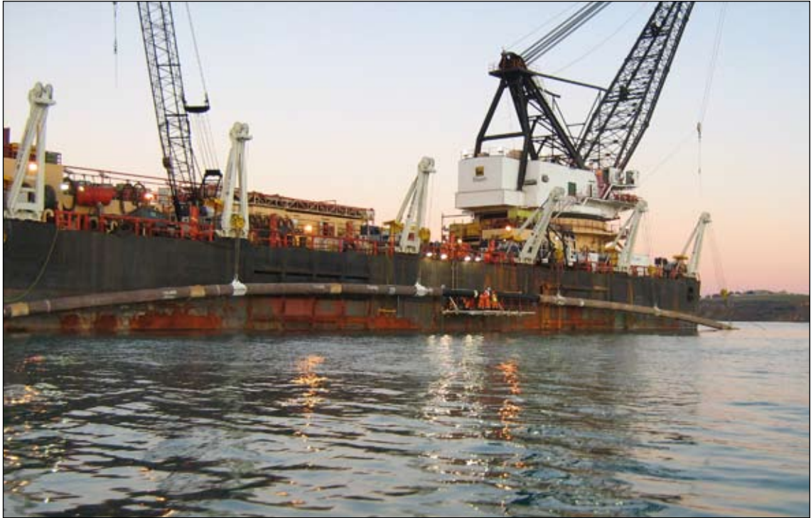
Final welding being carried out on the Medgaz pipeline, which was laid in 2008 and is currently being commissioned.
