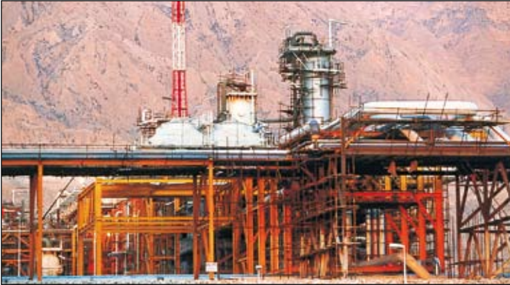
This plant in Assaluyeh treats gas from the South Pars field. Assaluyeh is also the origin of the IPI pipeline.
