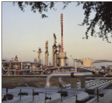
Natural gas processing unit - Guamaré, Rio Grande do Norte.
