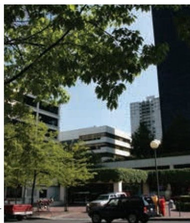
BELOW AND INSET LEFT No ugly external plant rooms at this building in the US city of Portland, Oregon (INSET LEFT), which is cooled and heated by this combined-cycle heat pump including a Capstone microturbine and a Yazaki 10 ton cooling unit (BELOW).
