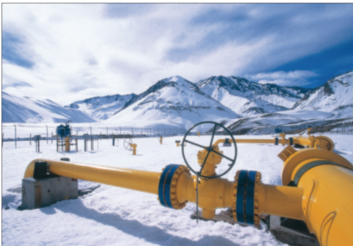
Argentina's gas resources include the world's most southerly production facility. This pipeline in Tierra del Fuego collects gas from the offshore Carina and Aries fields operated by Total in a consortium with Pan American Energy and Wintershall.
