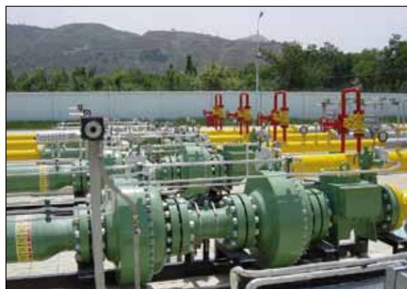
Gas pressure regulating station, China
