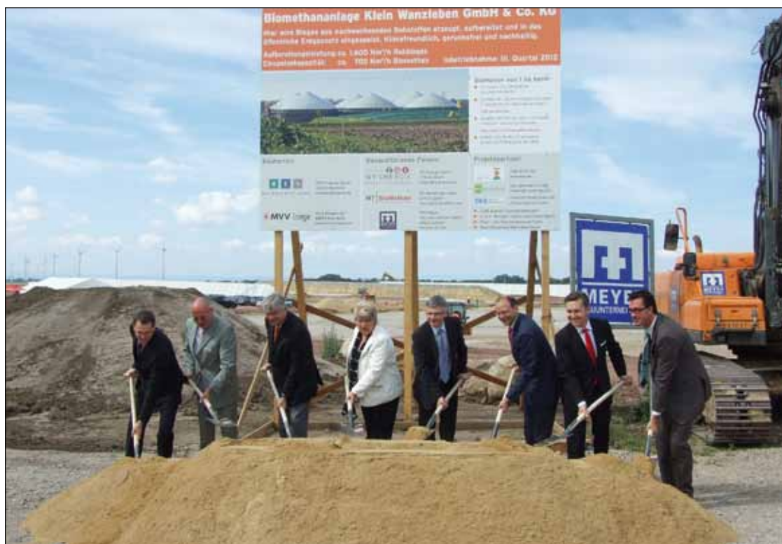
Breaking ground for a biomethane plant in Klein Wanzleben, Germany – the injection of non-conventional gases reduces the carbon intensity of the gas grid.
