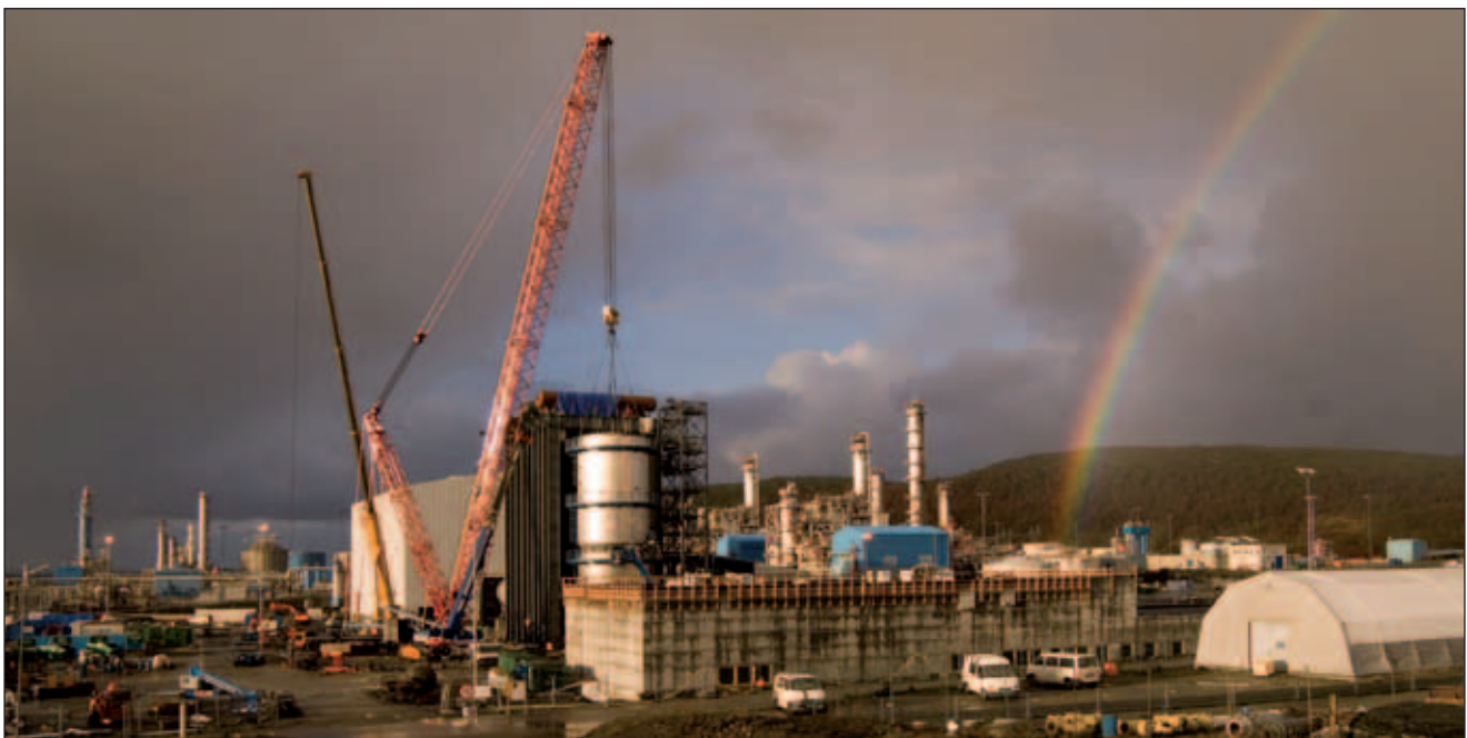
The Eurogas-Marcogaz LCA covers all steps of the natural gas chain – a gas-fired combined cycle power plant under construction in Kårstø, Norway.
