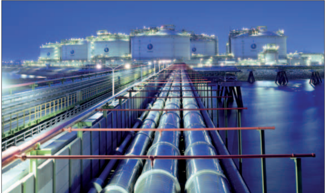
Korea has four LNG receiving terminals – this is Incheon which is operated by KOGAS – and plans to build a fifth by 2013.
