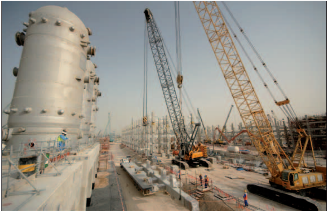
Work is well underway on Pearl GTL which represents an investment of over $20 billion.
