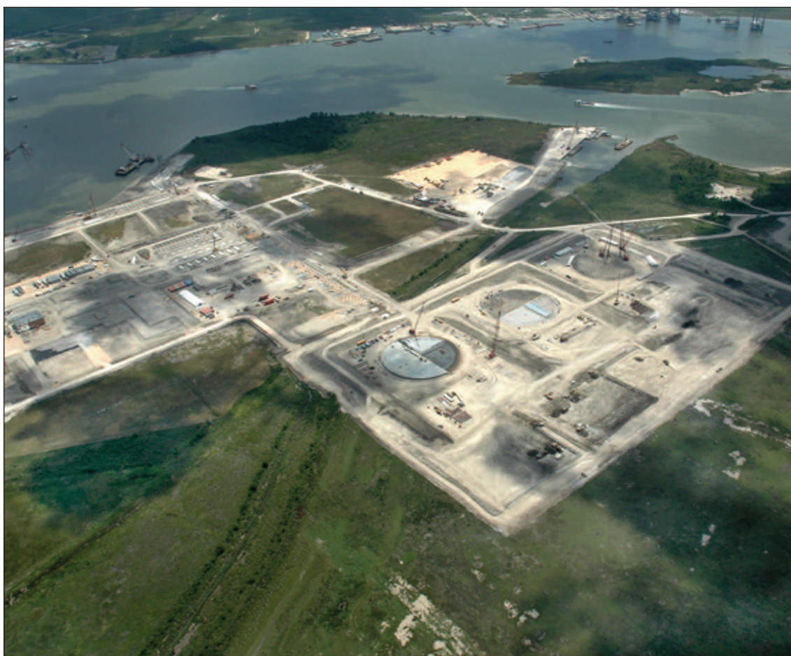
Bechtel has the EPC agreement for Cheniere's Sabine Pass LNG terminal and construction of the $820 million first phase started in March 2005.
