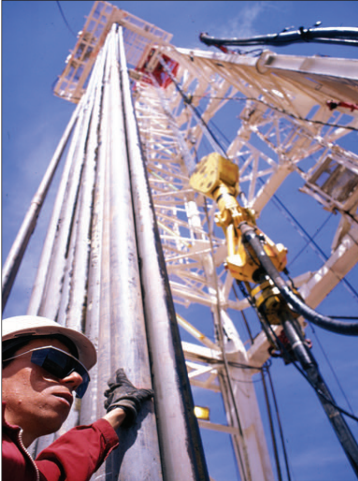
Gas drilling at In Salah – Algeria’s supply of gas to Europe is set to increase.
