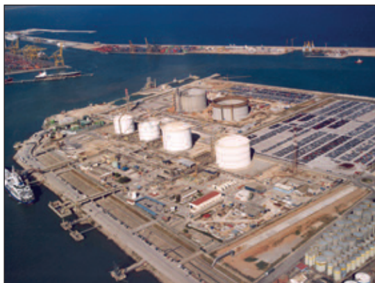
Spain’s first LNG regasification plant in Barcelona has been steadily expanded. A sixth storage tank is under construction.
