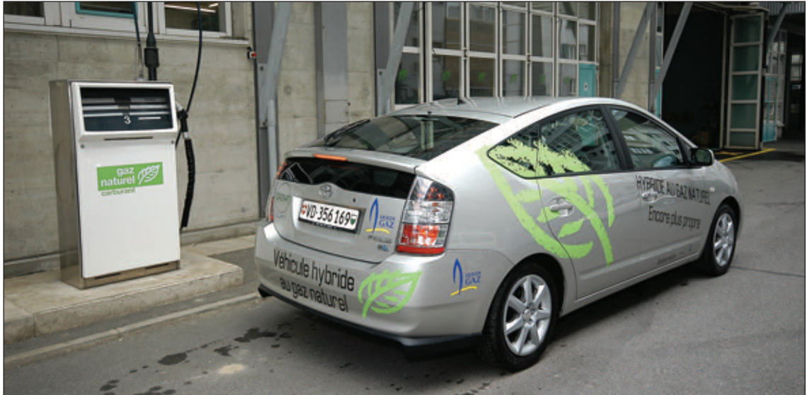
An NGV refuelling station at the Holdigaz headquarters in Vevey.
