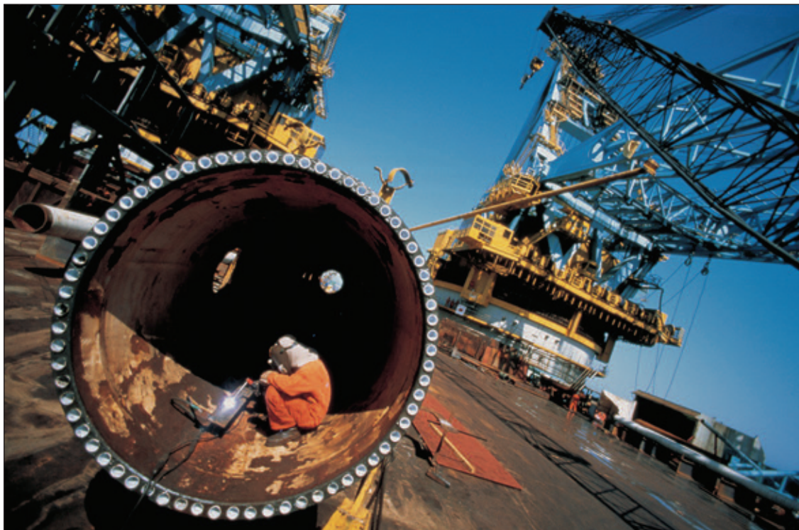
Laying the pipeline for the Blue Stream project connecting Russia and Turkey which was officially inaugurated in November 2005.
