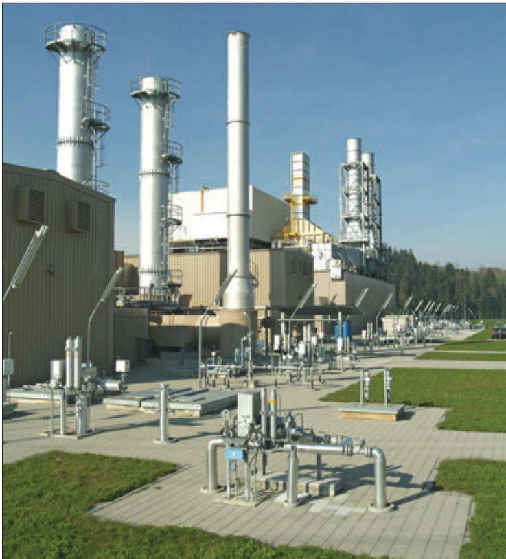
The compressor station at Ruswil (60 MW) is the operational centre of the Transitgas system.
