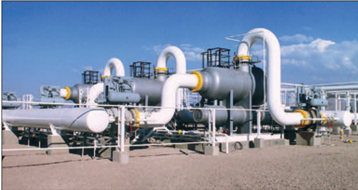
The Bazargan metering station on the border with Turkey.
