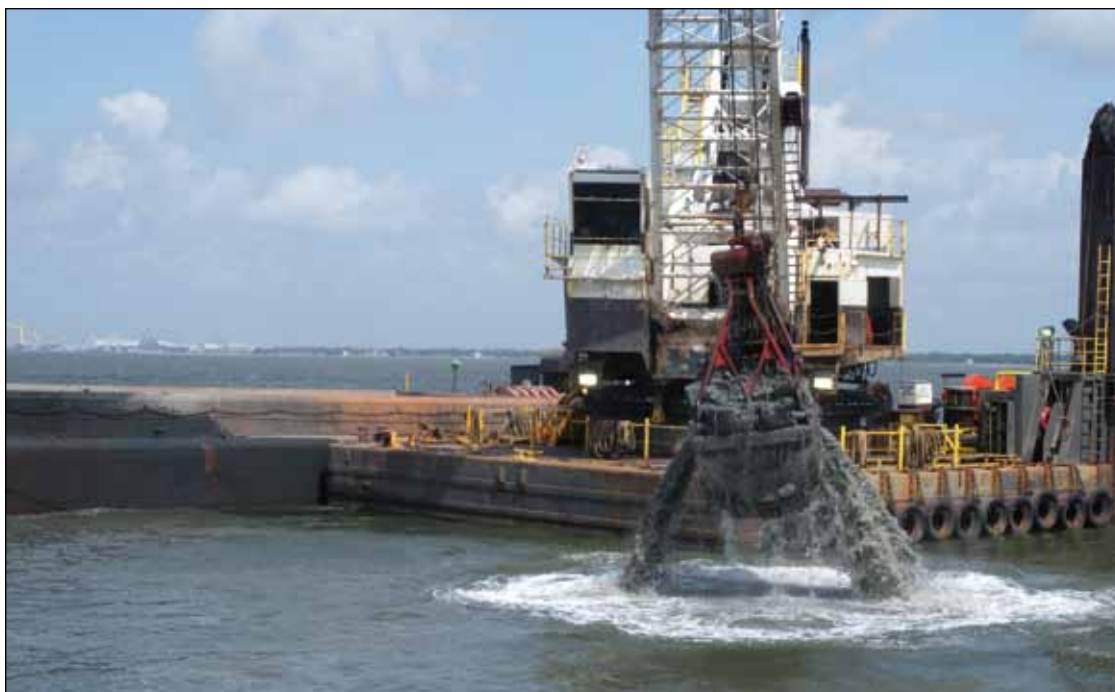
Dredging operations underway for the Gulf LNG receiving terminal in Pascagoula, Mississippi.
