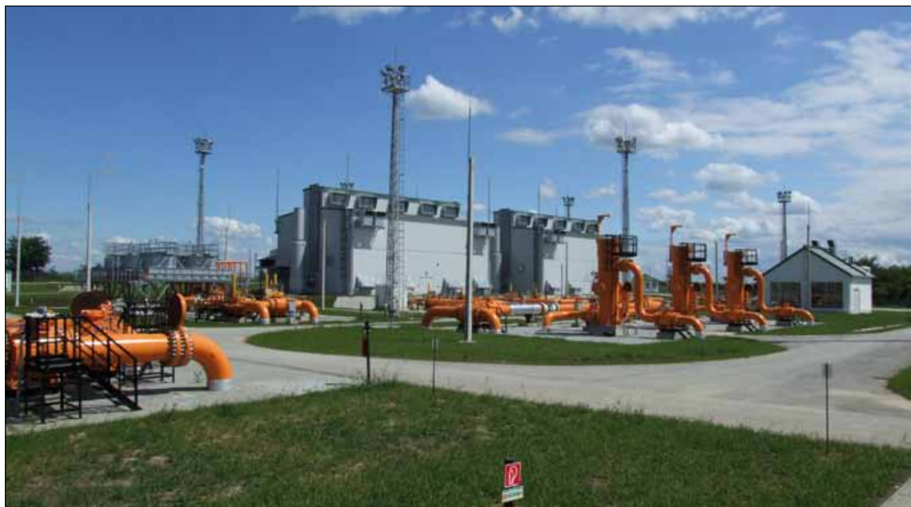
The Bata compressor station in Hungary on the Croatia-Hungary Gas Interconnector.
