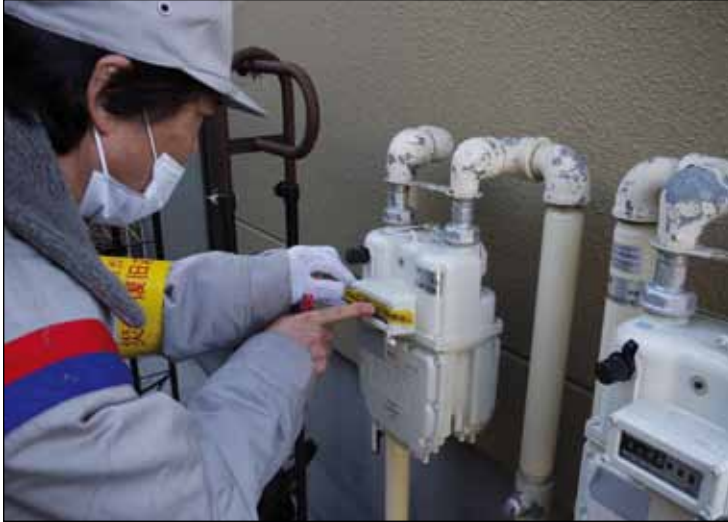
After the devastation of March, the smart gas meters which shut down automatically had to be carefully inspected.
