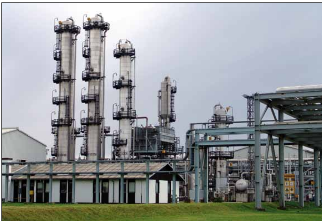
The gas treatment plant at the onshore Molve field.
