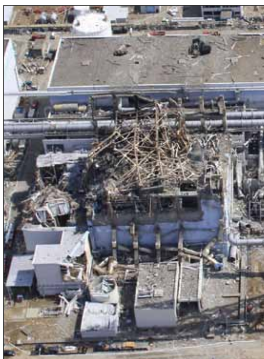
An aerial view of the Fukushima Daiichi Nuclear Power Station is a stark reminder of the destruction. Stabilisation work at the plant continues.
