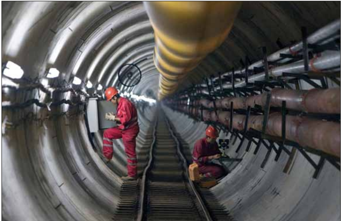
China has inaugurated the Second West-East Gas Pipeline as part of its plans to achieve long-term energy supply security.
