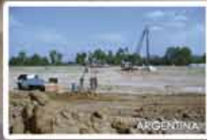
WATER PURIFICATION PLANT WATERS OF PARANA RIVER ARGENTINA
