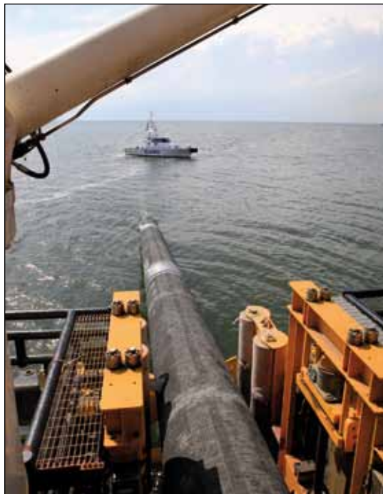
The first Nord Stream pipeline is due to open later this year.
