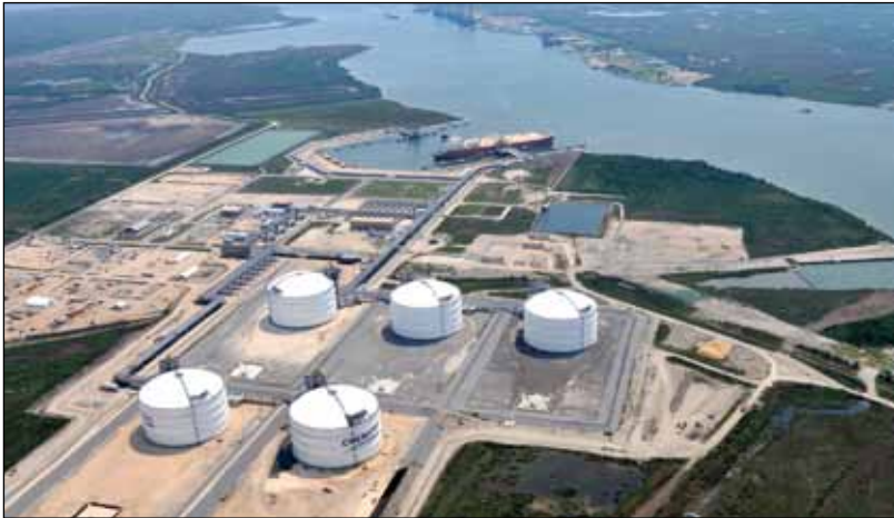
▲ Sabine Pass is the world's largest regasification terminal with a capacity of 113 mcm/day and is adding liquefaction trains for export.
