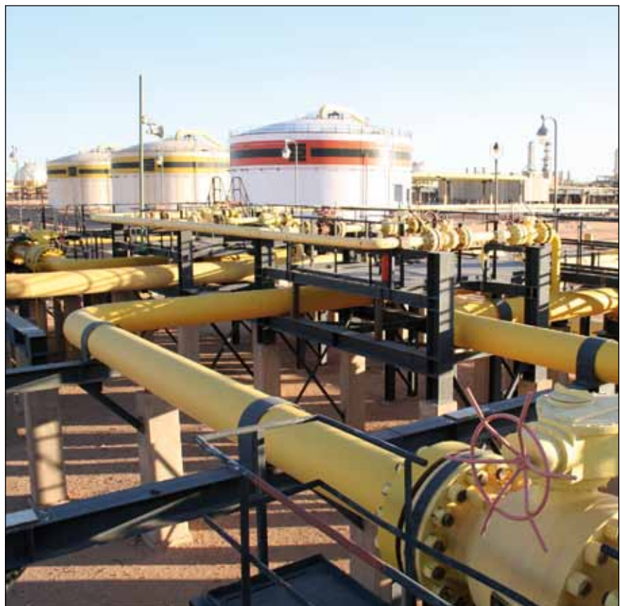
Hassi R'mel gas production facility.
