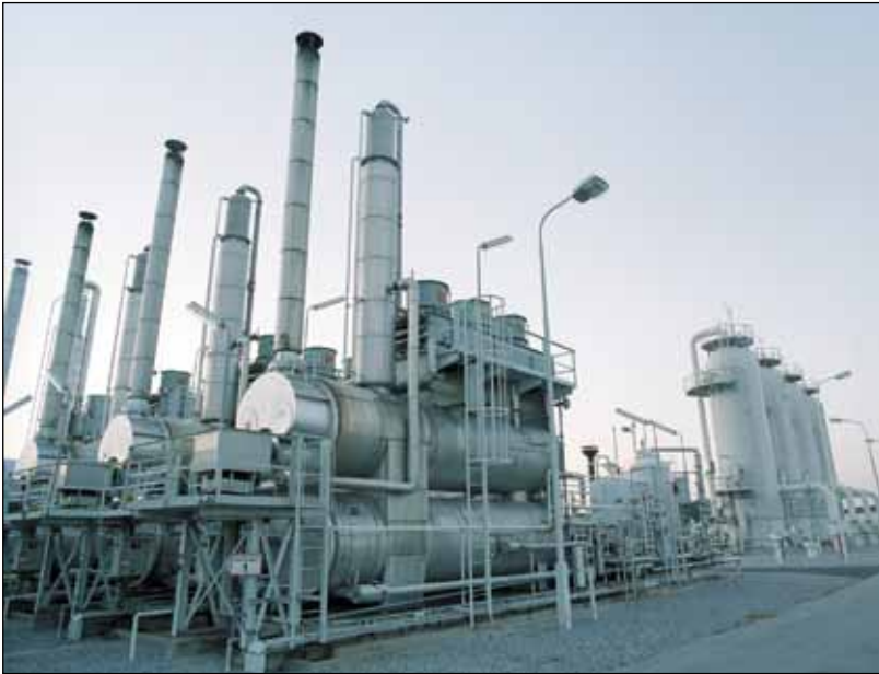
▲ The Baumgarten compressor station is an important distribution hub for Europe.
