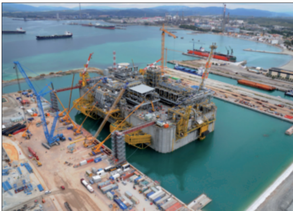
Qatar's involvement along the entire LNG chain includes a 45% stake in Italy's new offshore regasification terminal, Adriatic LNG, which is seen here being fitted out and is due to start operations by the end of 2008.
