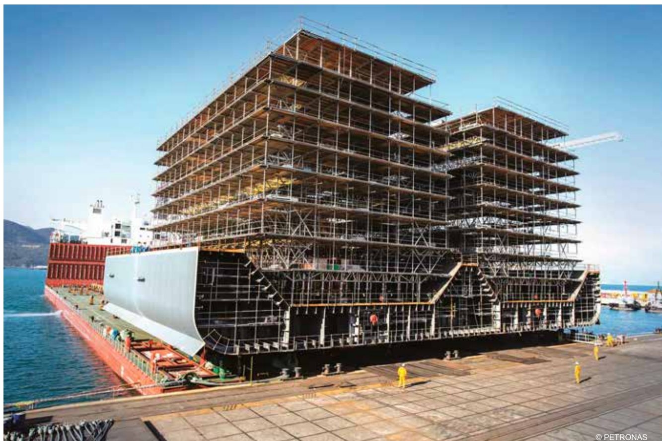
PETRONAS FLNG to be commissioned in 2015
