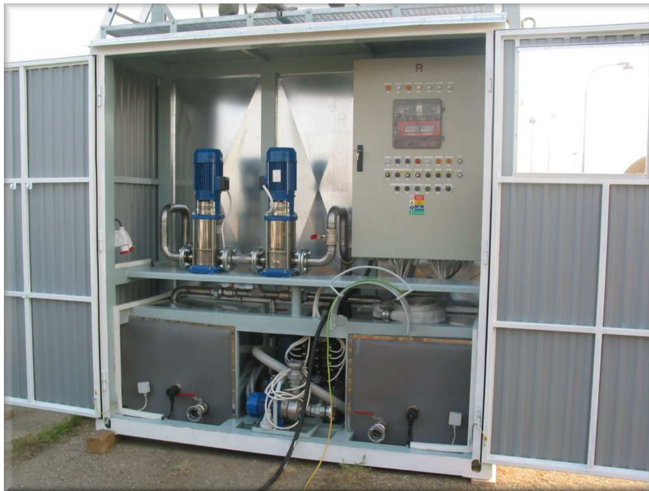
Unit Control System
