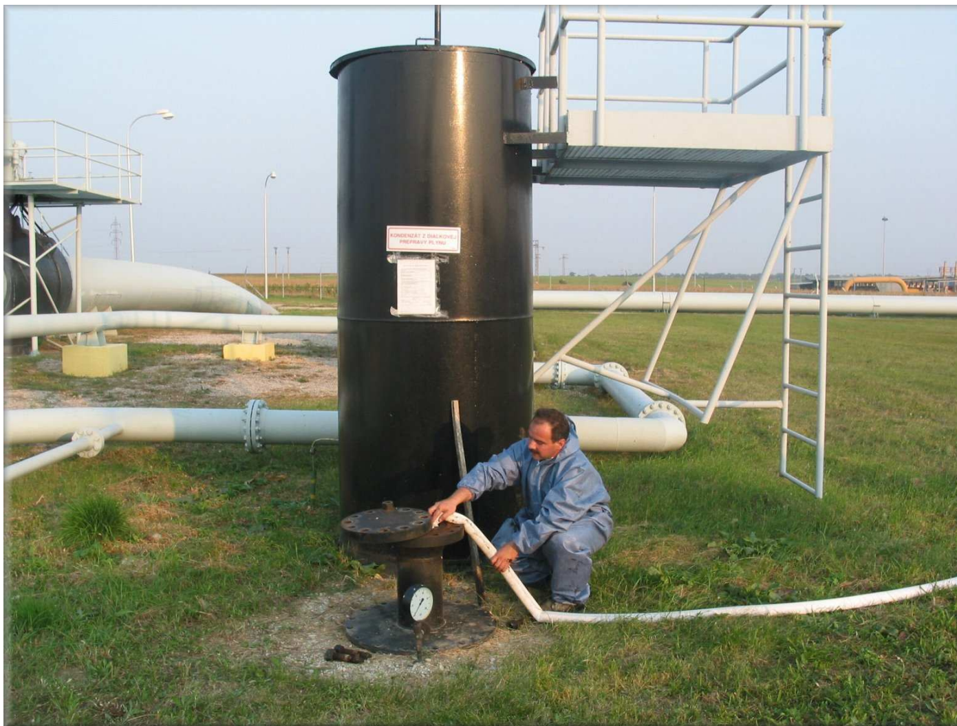
Waste release into the collecting tank
